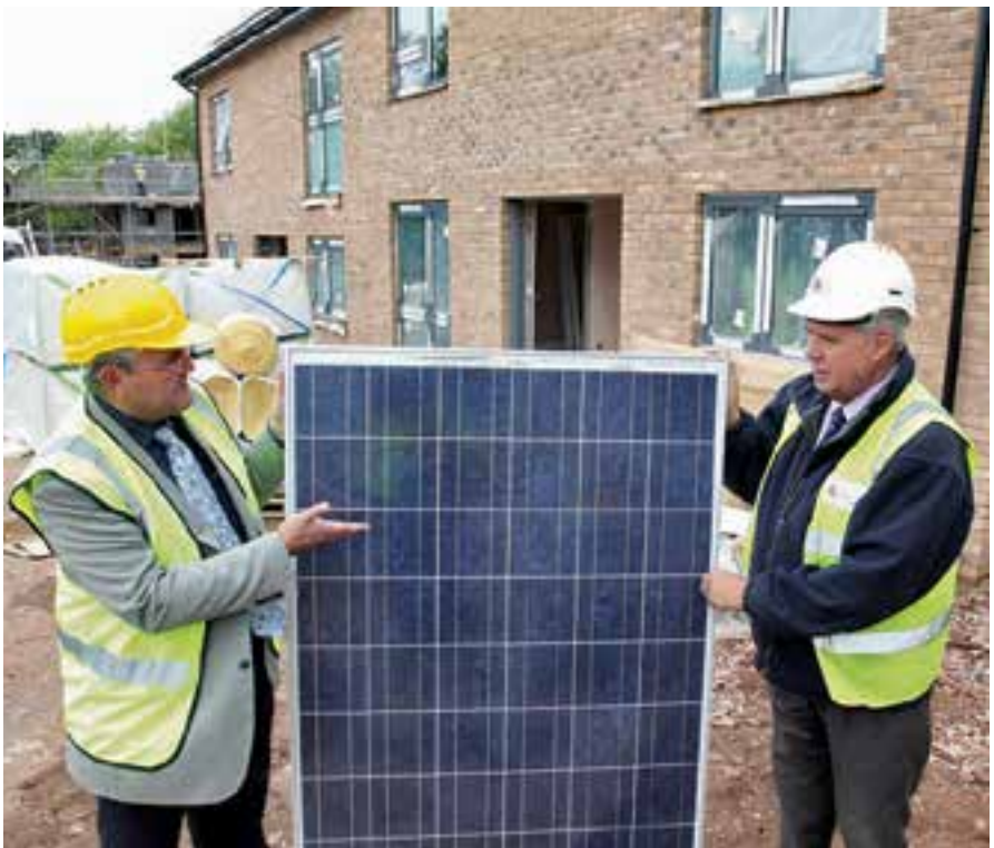
New housing with solar panels
