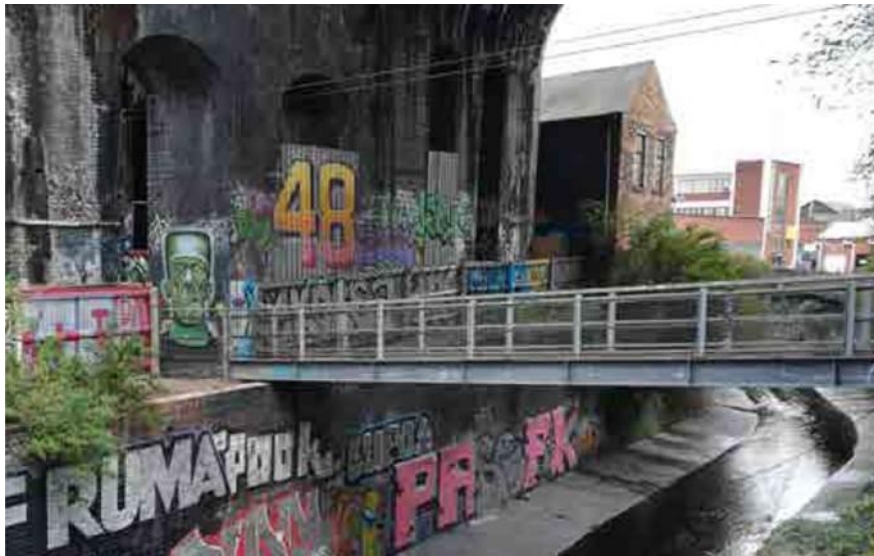
Fig 40: Existing Bridge Crossing River Rea below Bordesley Viaduct (to be Replaced) with Plot (CF2) to be redeveloped as Custard Factory Living in Background
